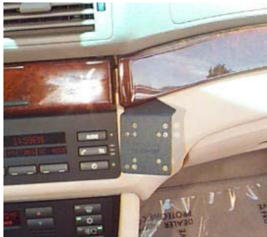
Finished Install Picture
